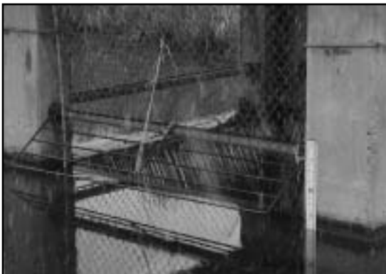
Brookhurst Dam Outlet
